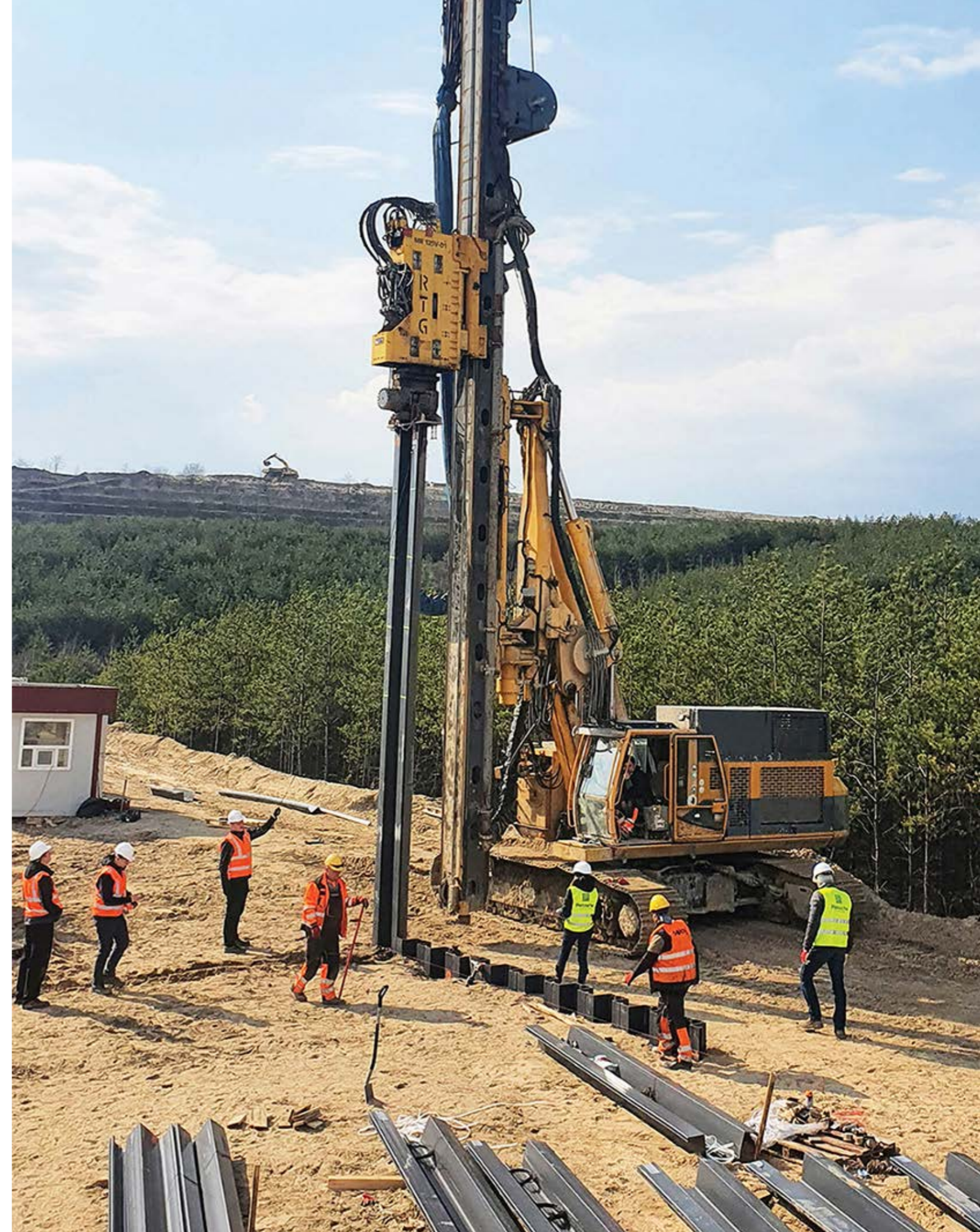
THE OLKUSZ AREA, POLAND: DRIVING OF THE SUPERLOCK HYBRID SHEET PILES IN ADVERSE SOIL CONDITIONS.
