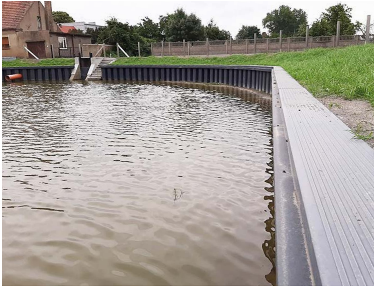
THE POZNAŃ AREA, POLAND: REVITALIZATION OF A WATER RESERVOIR - EMBANKMENT STABILIZATION WITH A VINYL SHEET PILING PALISADE FINISHED WITH A CAP AND MODERNIZATION OF WATER DISCHARGE BY INSTALLATION OF MODULAR VINYL SLUICE IN THE EXISTING WEIR.
