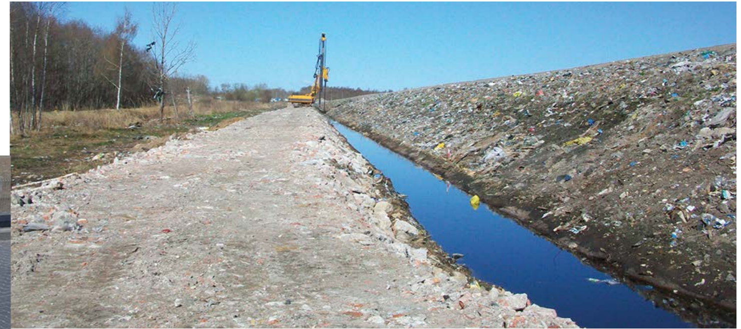
PARNU, ESTONIA: INSTALLATION OF A CUT-OFF WALL AT A TANNING FACILITY CHEMICAL WASTEYARD.
