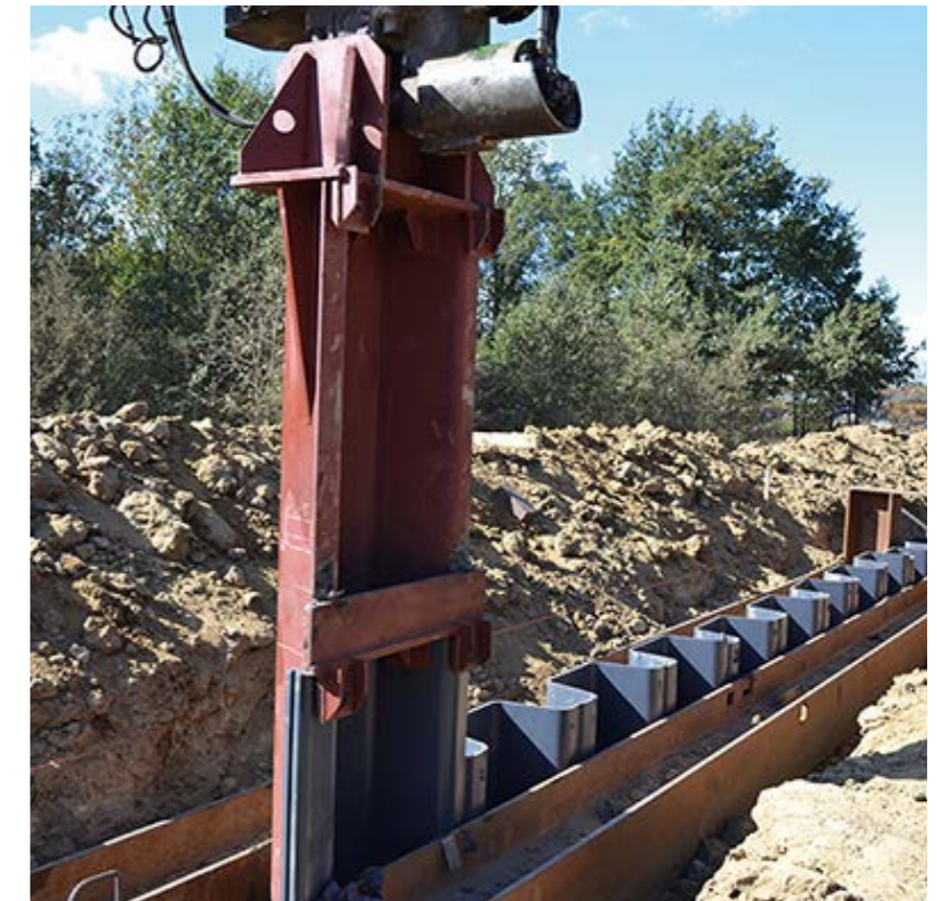
THE WROCLAW WATER JUNCTION, POLAND: REINFORCEMENT OF A FLOOD BANK WITH VINYL SHEET PILES - INSTALLATION WORKS.
