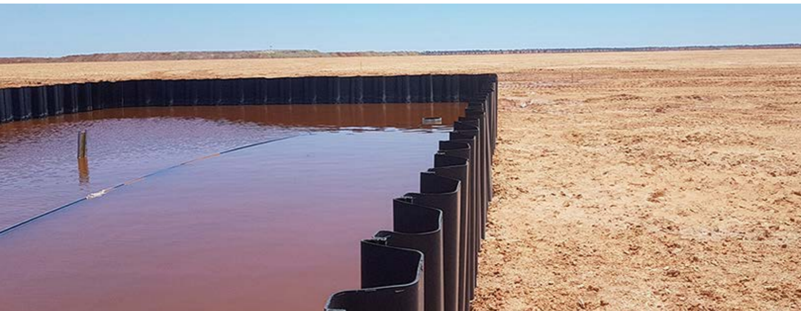
WILUNA, AUSTRALIA: BRINE RESERVOIR CONSTRUCTED USING VINYL SHEET PILES WITH INTEGRATED GASKETS MADE OF SOFT PVC.
