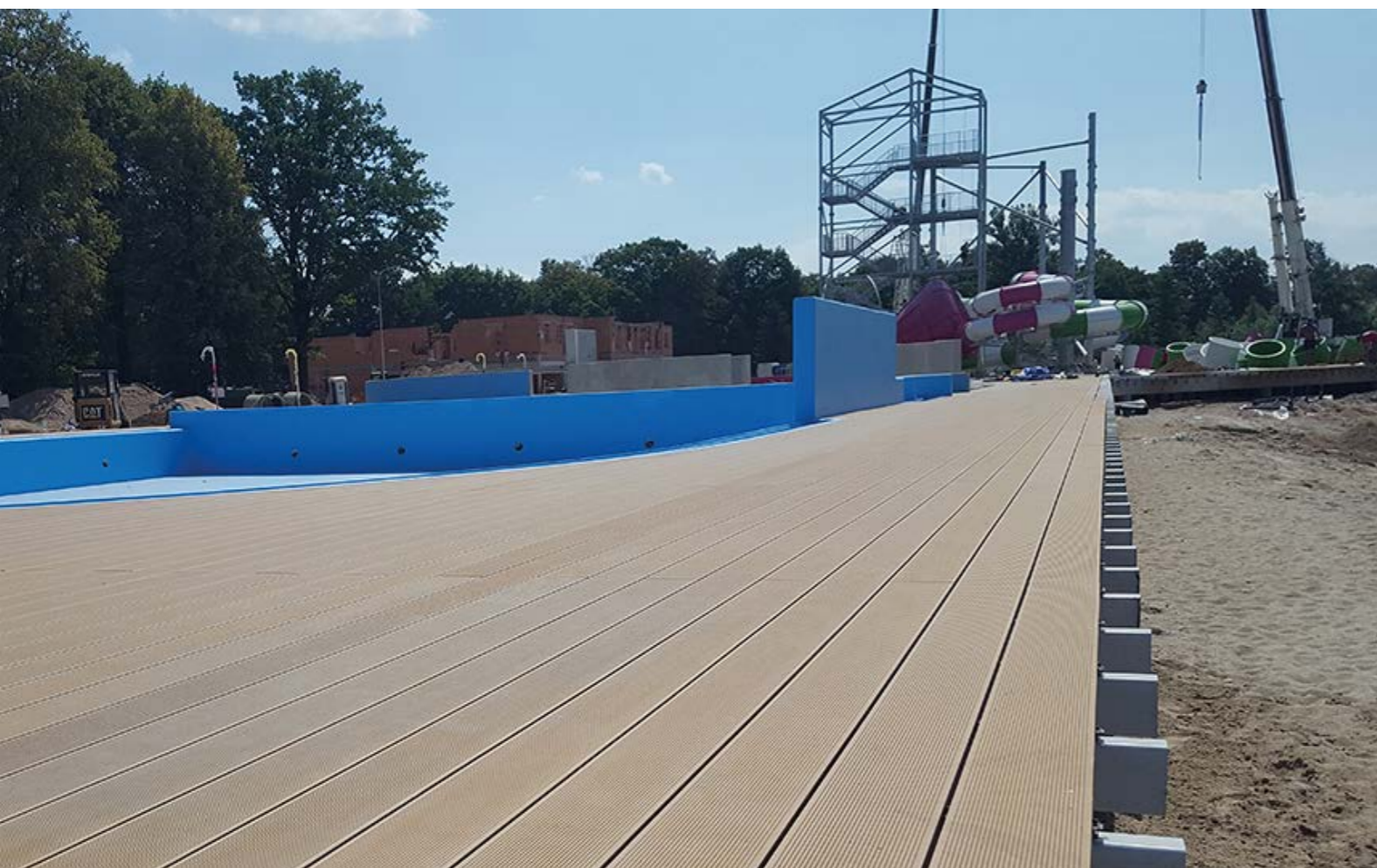
IN THIS PROJECT, APART FROM THE ECOLOCK VINYL SHEET PILING, THE TERRADECK COMPOSITE PLANKS WERE USED.
