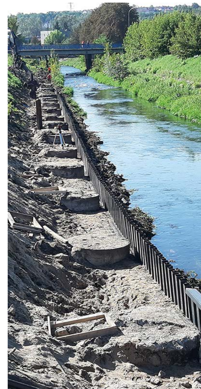
BĘDZIN, POLAND: DEVELOPMENT OF THE BOULEVARDS OF THE CZARNA PRZEMSZA RIVER ALLOWING FOR THE CONSTRUCTION OF A MARINA.
